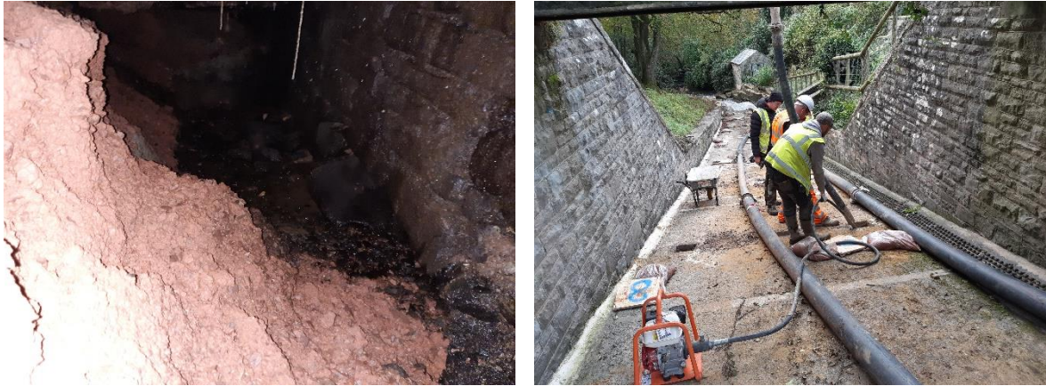
Picture 1 & 2 ©Forestry England - Left - example of voids found beneath spillway. Right - grouting undertaken to make safe in short-term.
